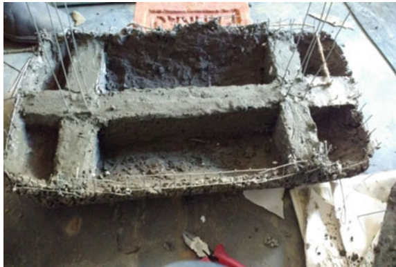
Fig. 3 Modified footing with voids inside
